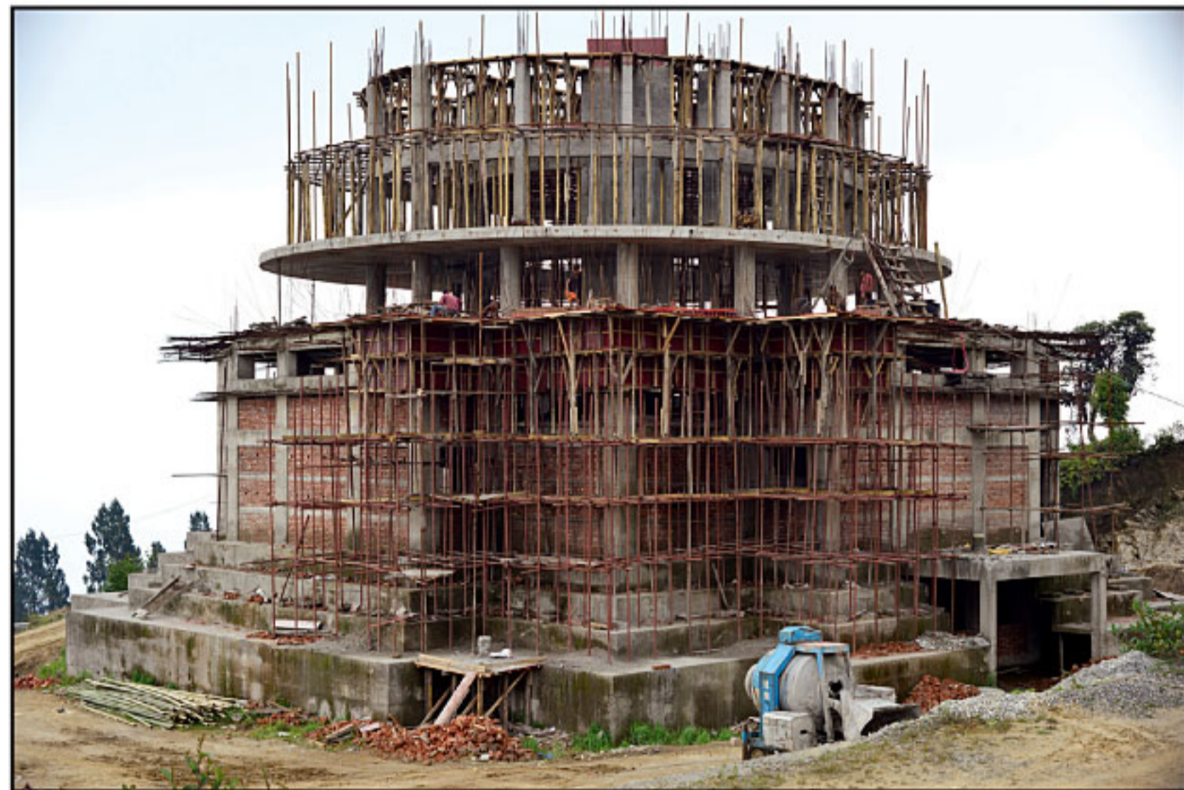
A recent picture of the under-construction Chenrezig Shingkhom project. (Next Buildings & Housing senior architect Gary Chapel giving a presentation on Chenrezig Shingkhom project at the project site.
